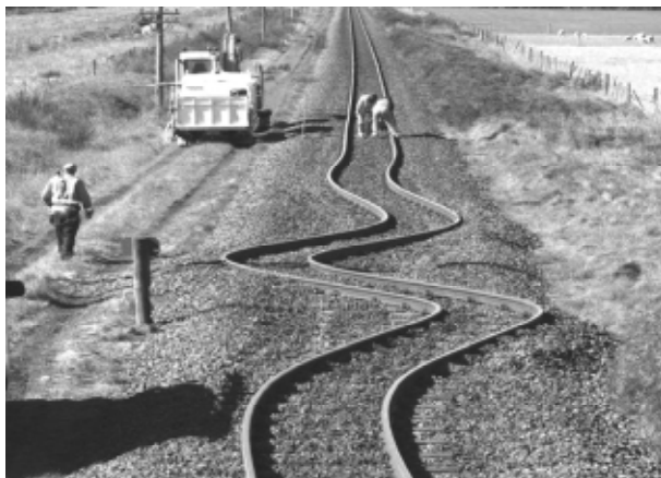
Figure 5. Photograph of a buckled track from www.modernghana.com/news/305521/1/earthquake-twists-railway-tracks.html .
