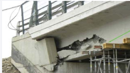
Seismic damage to shear key and abutment
