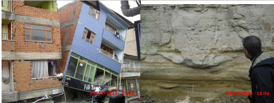
ERCIS: The Thick soft soil Deposits amplified the ground shaking and damages.
