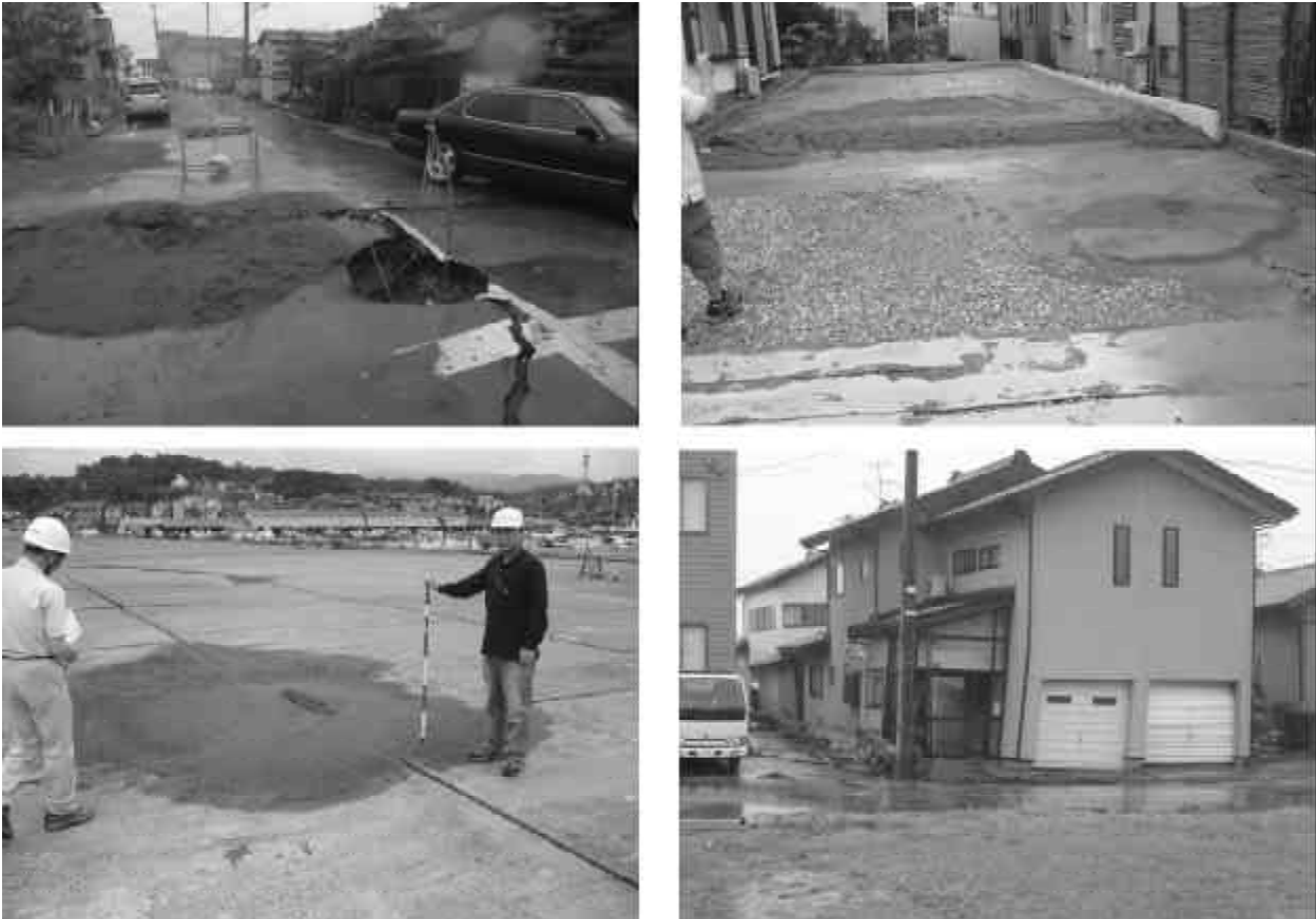
Figure 10. The liquefaction observed at Matsunami 2 in Kashiwazaki city that cause damage to utility poles, asphalt roads and foundation of houses.
